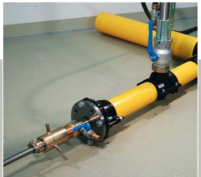
Picture 5: Drilling via AQUAFAST® clamp flange and FRIALEN® SPA shut off saddles with setting device
